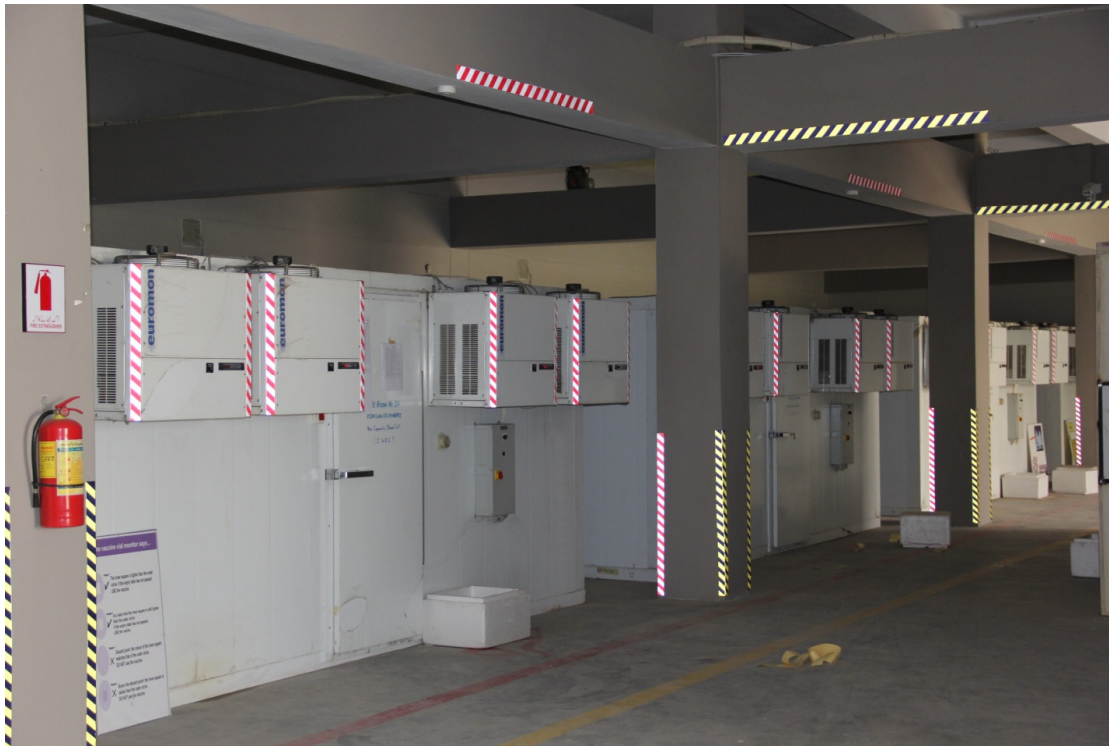
Figure 19. Cold Room 50 m 3 Capacity at Store
